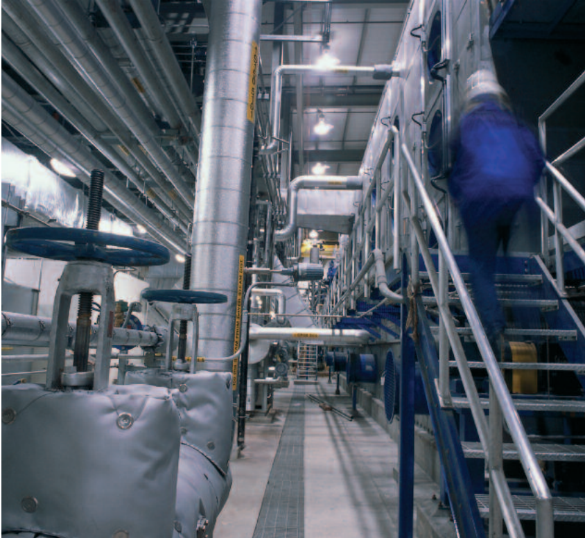
Plant control solutions
